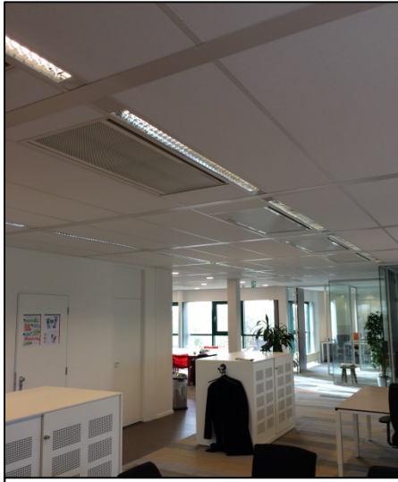
CBM in a straight line in a Dutch office building
