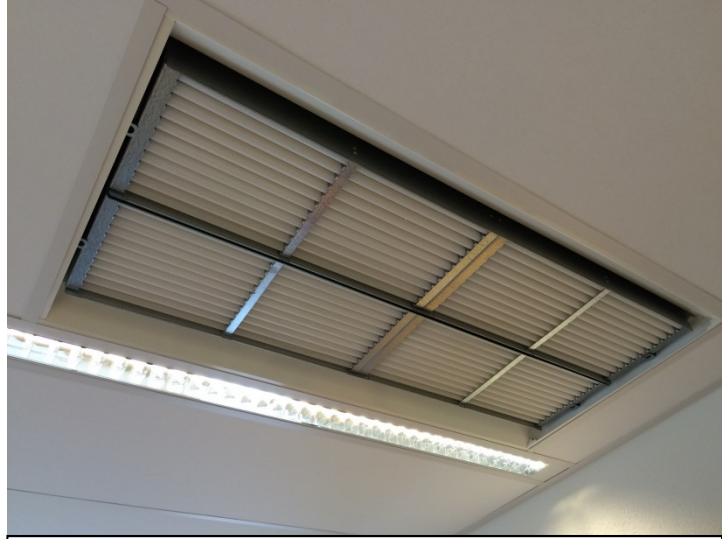
The thermal PCM battery made from HDPE panels filled with a phase change material
